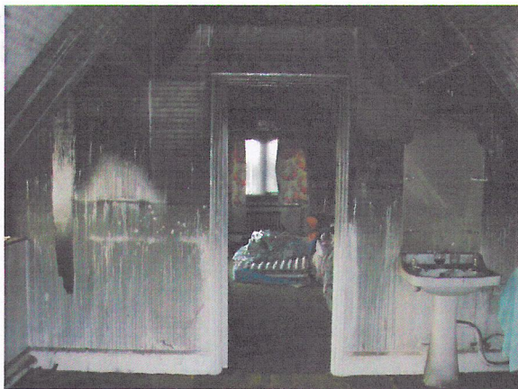
Heat & Smoke Damage - Top of Room
