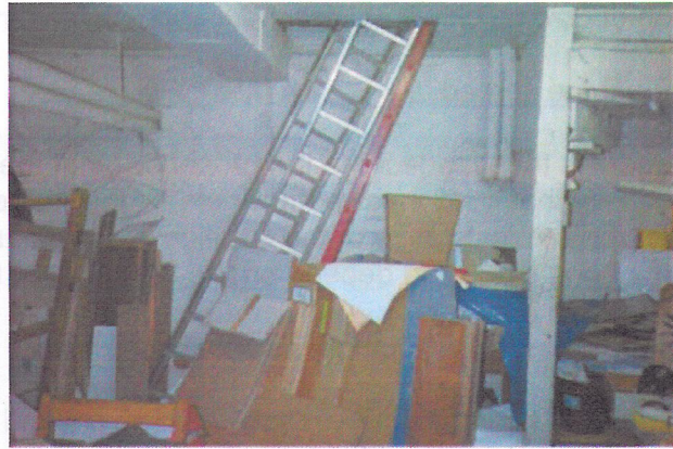
Basement High Fire Load & Access Problems
