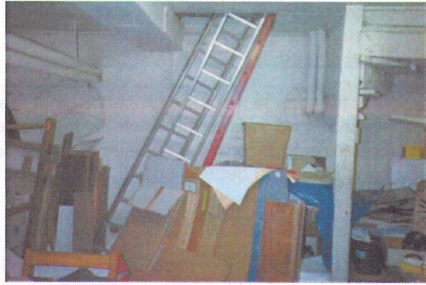
Basement High Fire Load & Access Problems
