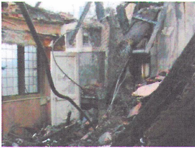
Debris Collapsing onto Lower Floors
