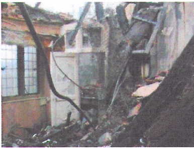
Debris Collapsing onto Lower Floors
