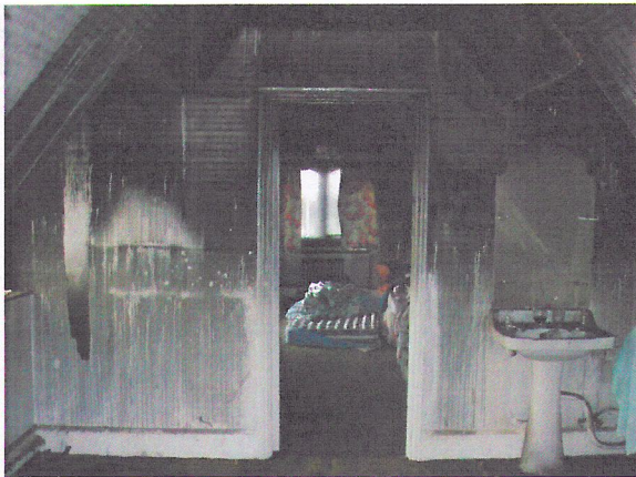
Heat & Smoke Damage - Top of Room
