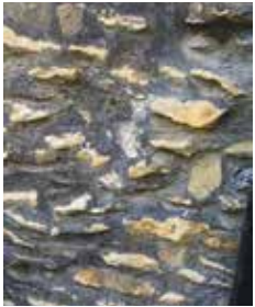
7. Both the outer and inner walls of Old Court were faced in randomly-laid Barnack ragstone. The original golden-yellow colour can be glimpsed here through the sooty weathering
